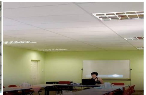
Suspended Ceiling Vinyl Faced Board 600mm x 1200mm Board Room
