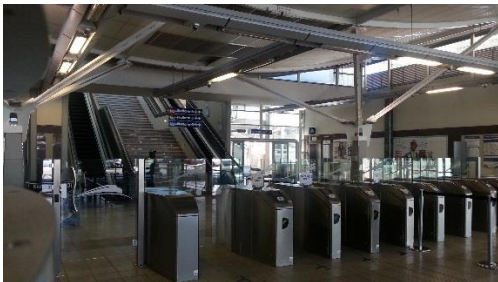
Suspended Ceiling Metroboard 600mm x 1200mm Railway Turnstiles
